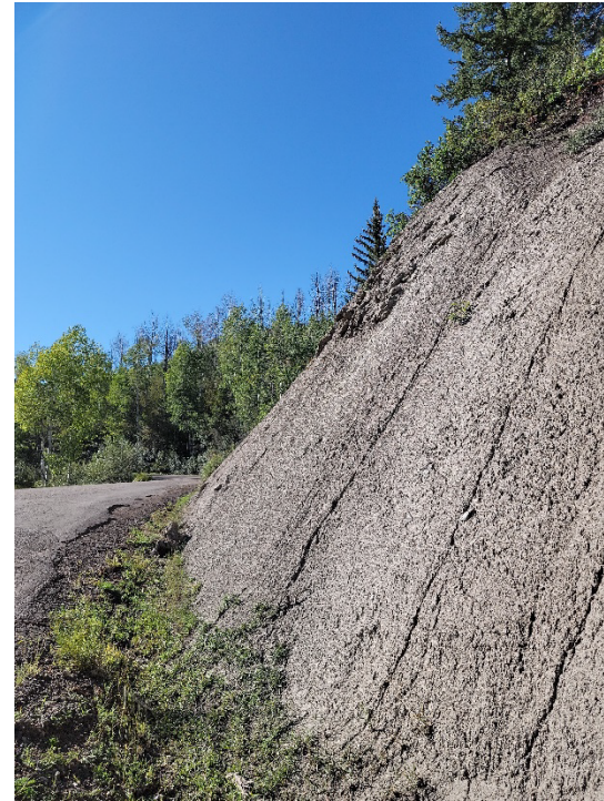
Photo 6. Closer look at steep slope surficial conditions. Note the erosion from surface runoff.
