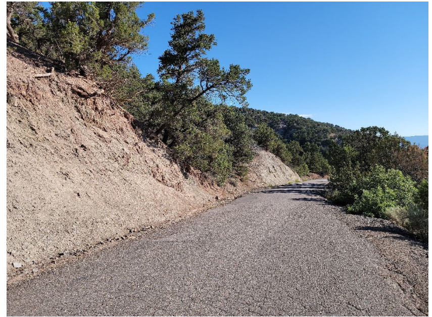
Photo 2. Steep slopes with weakly cemented surficial soils
